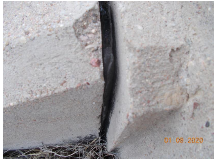
Suspect asbestos-containing material M-21-B-EJM01. The expansion joint material is non-detect for asbestos.
