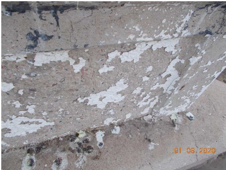
Paint sample M-21-B-LP01. The white paint on concrete is considered lead-containing paint.
