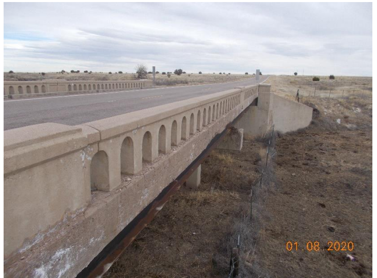
Paint sample M-21-B-LP02. The black paint on the metal girders is considered lead-based paint.
